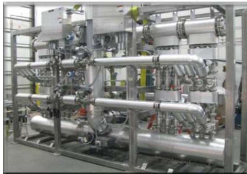
Pretreatment Processing Full Scale Rig Ethanol Production Plant, USA
